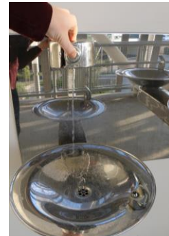
Innovation Building Water Bottle Fillers
